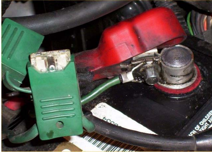
Figure 2- Top post battery connection & fuse holder
